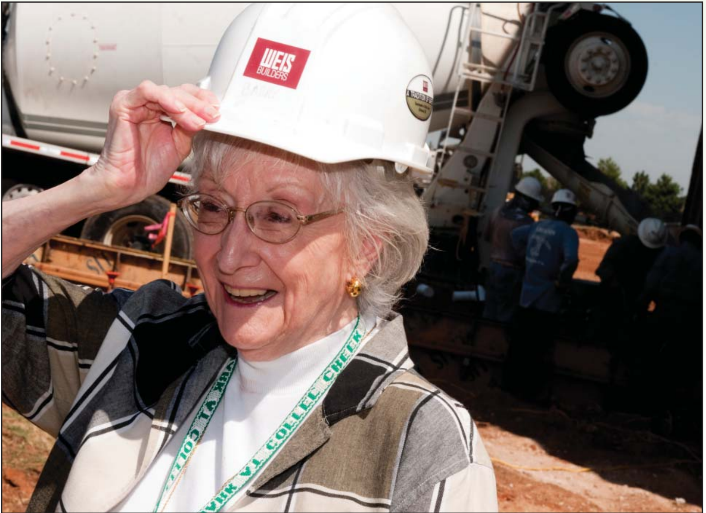
Marion Maier shows her excitement at the recent groundbreaking for Touchmark's $15 million expansion, which will add 73,000 square feet to the community.
